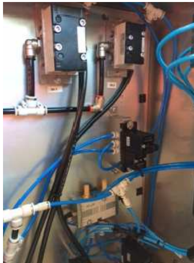
Pneumatics inside Control Box
